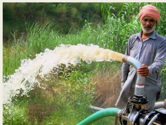
A solar water pump installation. Photo courtesy of Global LEAP Awards.
