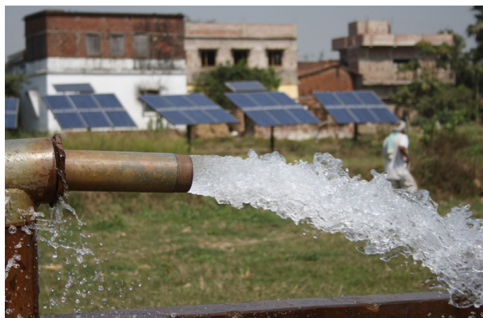
A multi-kilowatt solar water pump installation in India. Photo courtesy of Claro Energy.
