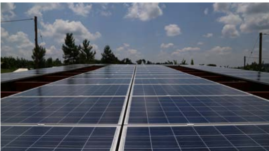
Top view of the Kanyegaramire mini-grid
